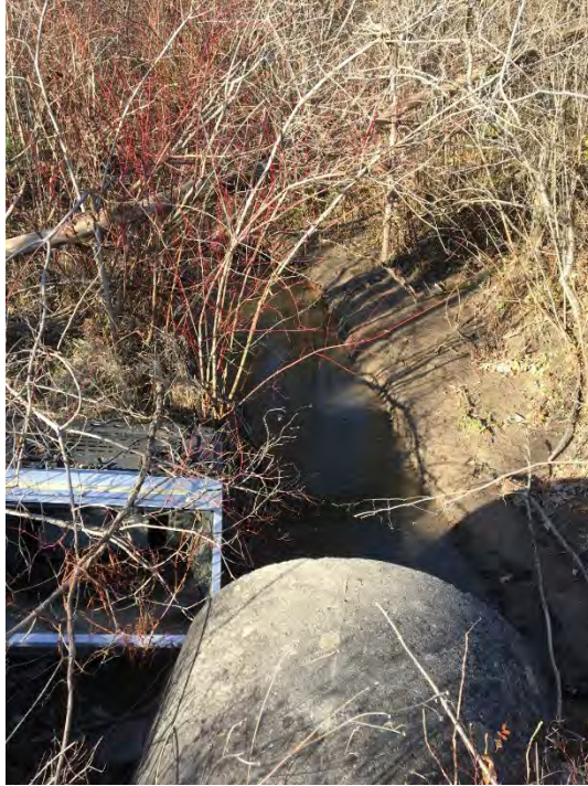
Photo 18: Looking north, inlet of the concrete pipe culvert conveying flow to the Welland River (November 2017).
