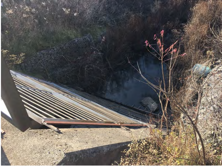
Photo 7: Looking southwest, at the outlet of the concrete siphon culvert beneath John Daly Way (November 2017).
