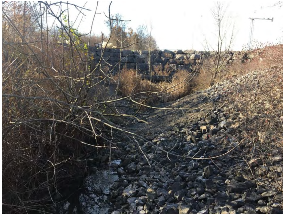
Photo 5: Looking southwest at the concrete siphon culvert through which the Conrail Drain flows, upstream of John Daly Way (November, 2017).
