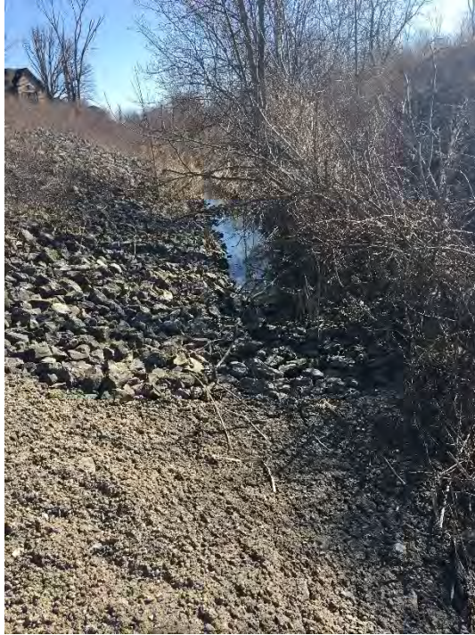
Photo 28: Looking north, the barrier to fish movement upstream of the syphon beneath John Daly Way (April 23, 2018).
