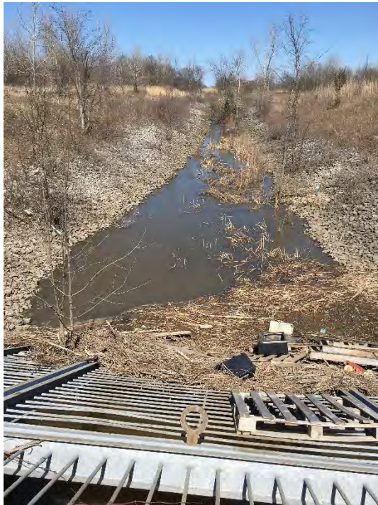
Photo 31: Looking north, the inlet to the culvert beneath Dorchester Road south of the Thundering Waters Study area (April 26, 2018).
