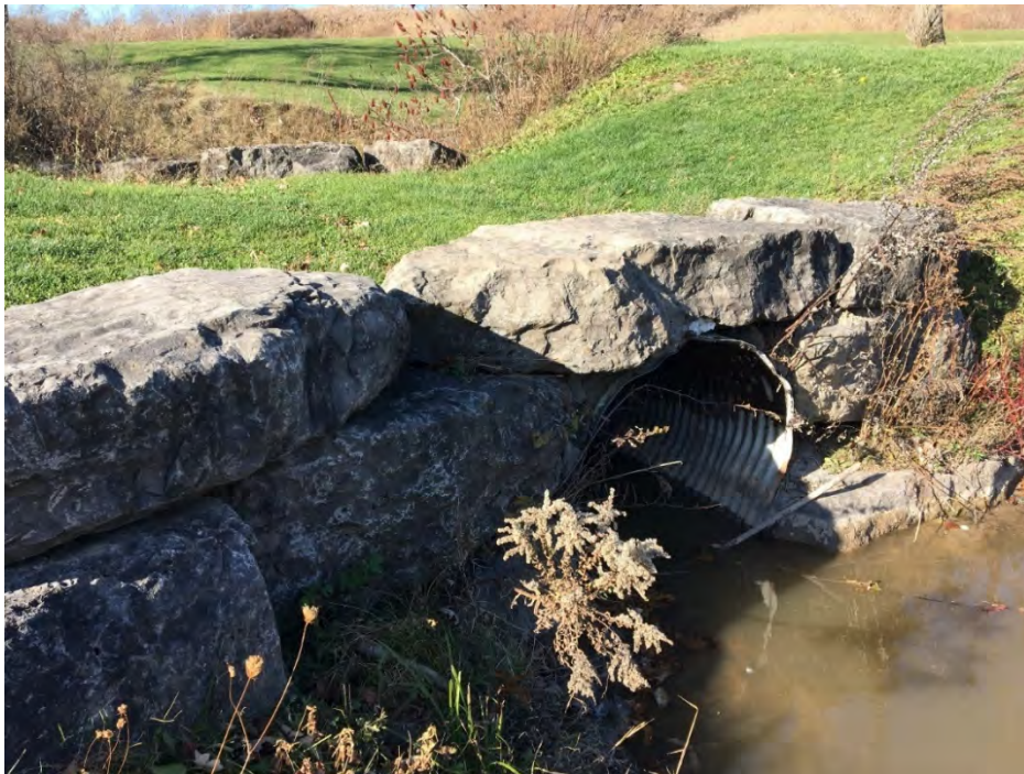
Photo 13: Looking south, water flowing through a corrugated steel pipe. Note, water level is at a level that it is conveyed through the CSP culvert (November 2017).
