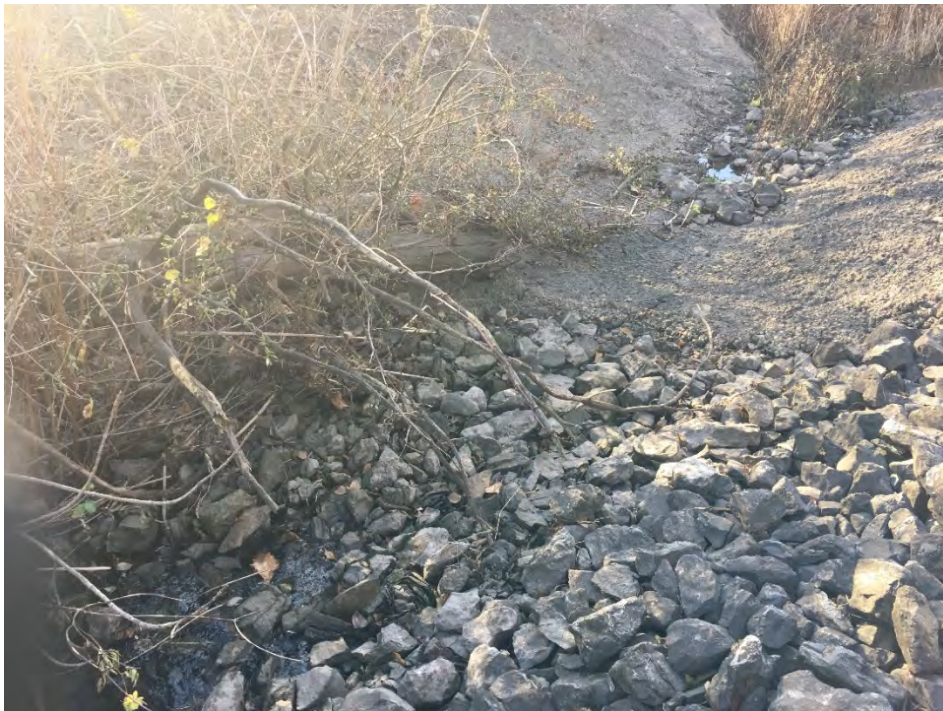
Photo 6: Looking southwest at the concrete/rip rap barrier upstream of the siphon culvert through which the Conrail Drain flows, upstream of John Daly Way (November, 2017).
