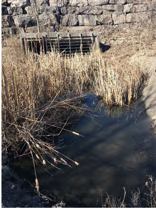
Photo 26: Looking south, the inlet of the syphon culvert beneath John Daly Way, downstream of the barrier to fish movement (April 23, 2018).
