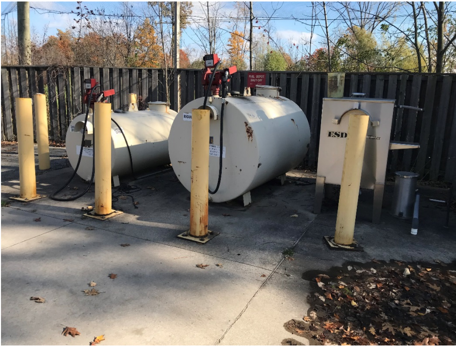
Photograph 5: Gasoline and diesel ASTs located on the northwestern portion of the Site.
